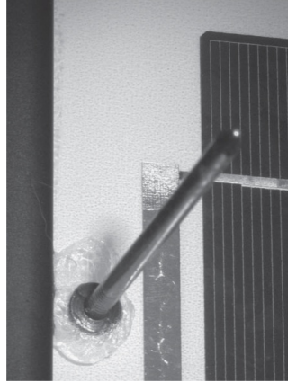
An example of using the nail test to correctly angle a panel
