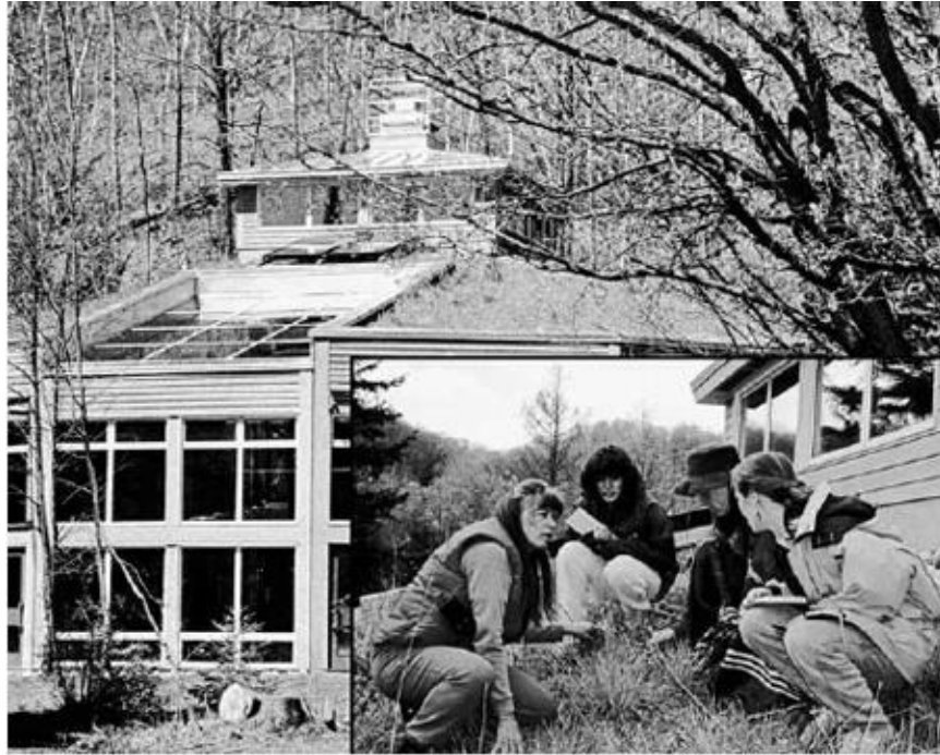
Students inspect a sod roof at the Boyne River School outside Toronto. Rain is held by the sod and released slowly, reducing storm surge. The runoff is clean enough to drink without treatment. [Credit: Peter Bane]
