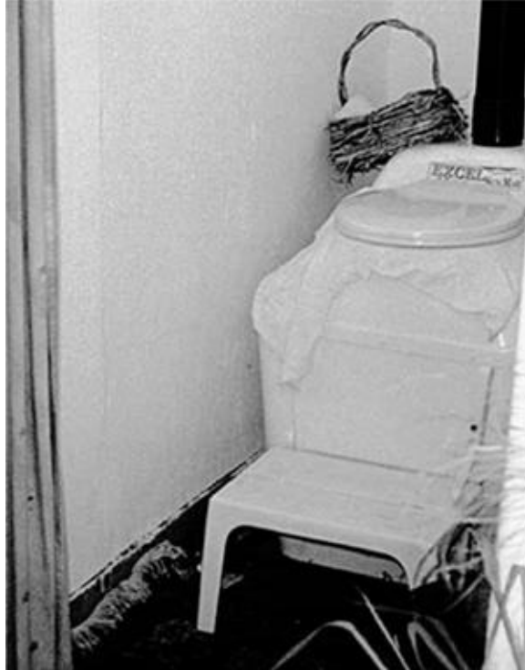
A Sun-Mar toilet installed in a California home. Note the black vent pipe. [Credit: Peter Bane]
