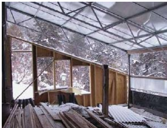
2. Construction of the new Phoenix greenhouse shows a main adaptive strategy for the challenging climate on Basalt Mountain. [Credit: Jerome Osentowski]
