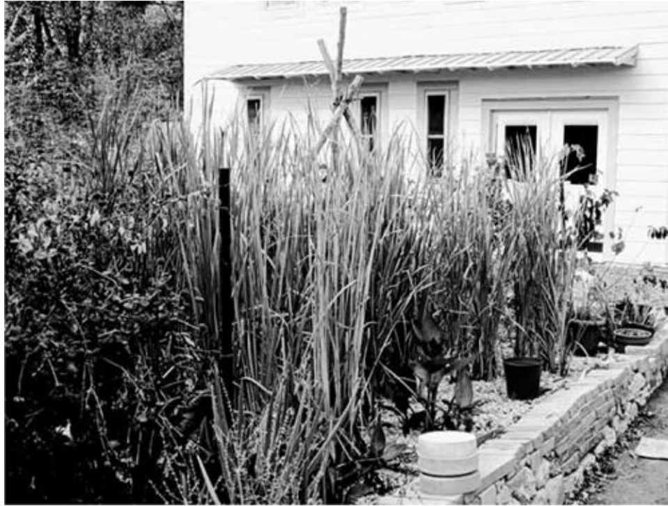
This wetland cell is populated by cattails and cannas. They grow out of the gravel medium with their roots in the subsurface wastewater. [Credit: Creighton Hofeditz]
