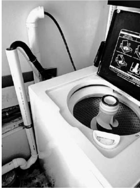
Two drain pipes and a flexible drain hose offer most householders the option to move laundry greywater to a biofilter trench or into septic lines for conventional treatment. [Credit: Creighton Hofeditz]
