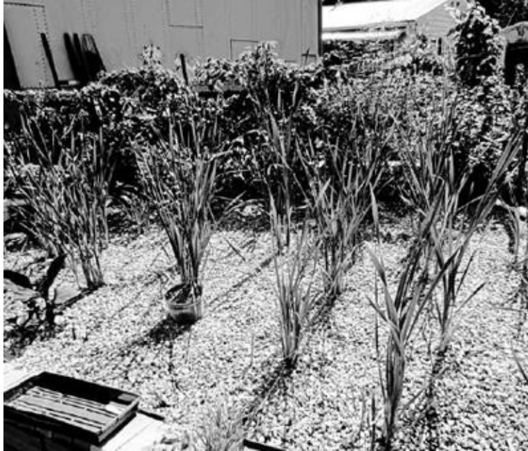
A wetland water treatment cell showing cattails emerging from a gravel matrix. The cell is lined and in this case raised above grade level to facilitate outflow toward ponds. [Credit: Creighton Hofeditz]
