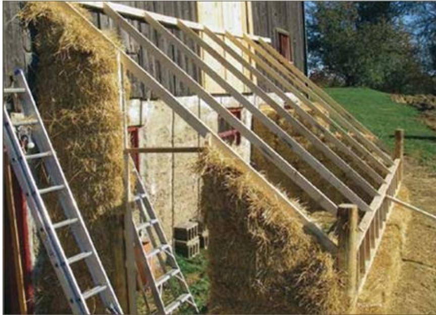
2. One of the first new constructions was this strawbale lean-to greenhouse against the south side of the barn. [Credit: Ian Graham]
