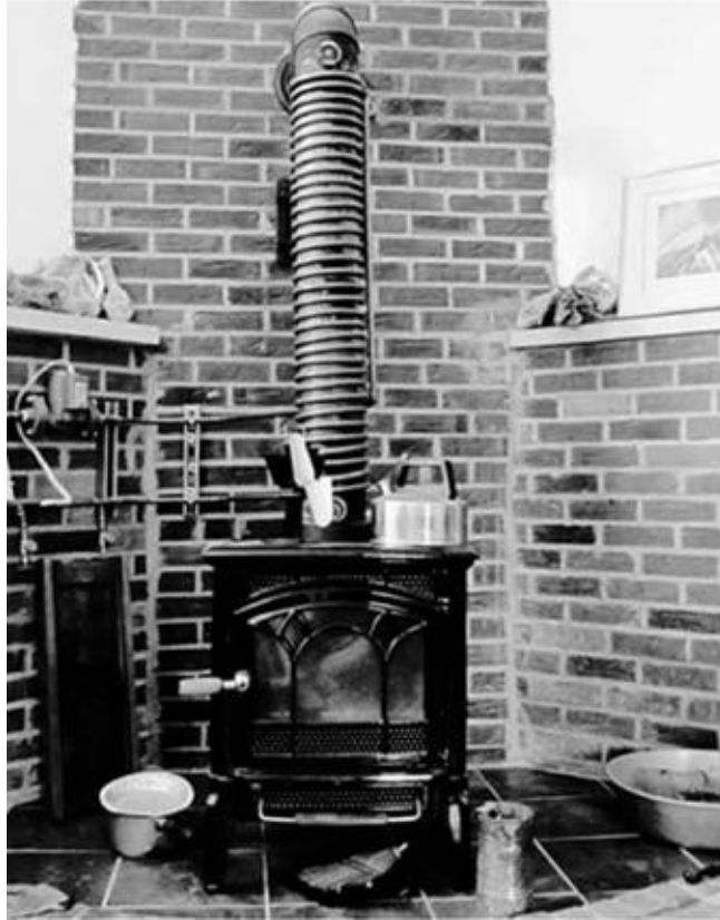
A resilient and economical home heating system supplied by local, carbon-neutral fuel. [Credit: Edward Carter]
