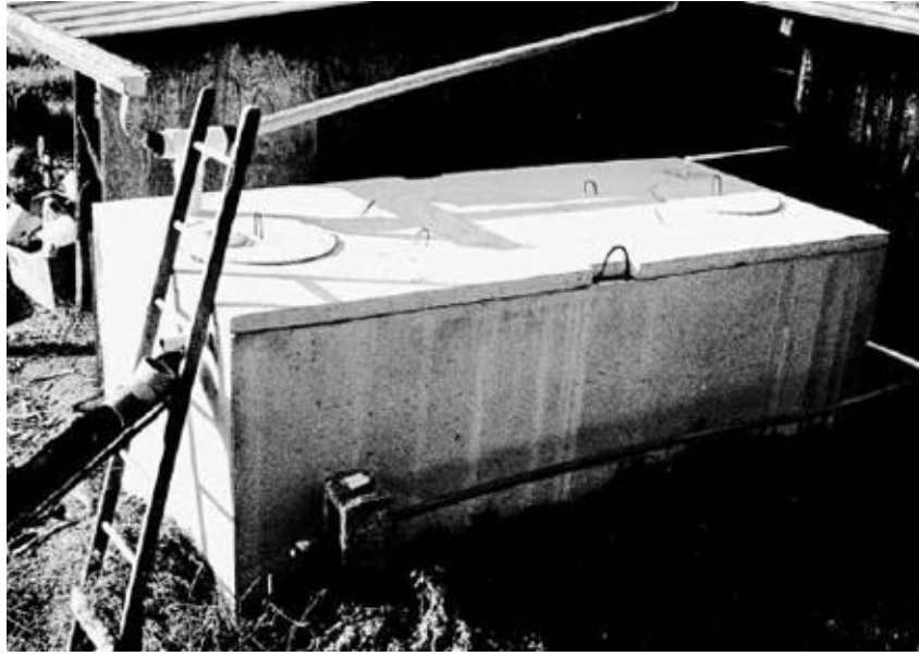
A precast concrete septic vault makes a fast and easy water tank. [Credit: Peter Bane]
