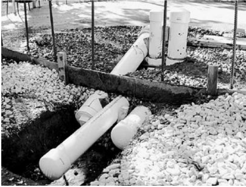
Three pipes positioned through the slab will provide inflow from gutters/standpipes, outflow to hydrants and a drain for cleaning the tank. [Credit: Keith Johnson]
