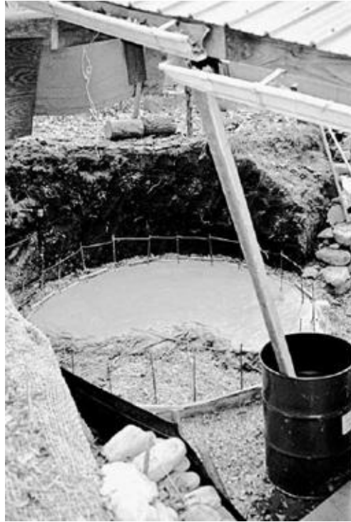
A 1,600-gallon ferrocement tank as its slab is being poured. A “spider” of rebar reinforces the slab and sticks up to form the lower reinforcement of the walls. All work on this small tank was done by hand, including concrete and mortar mixing. [Credit: Peter Bane]
