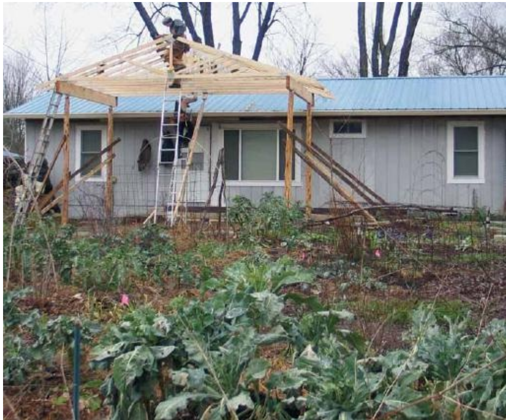
4. Taking advantage of mild autumn weather, we erected a new porch to carry solar panels, and to provide a dignified entry and outdoor room. [Credit: Peter Bane]
